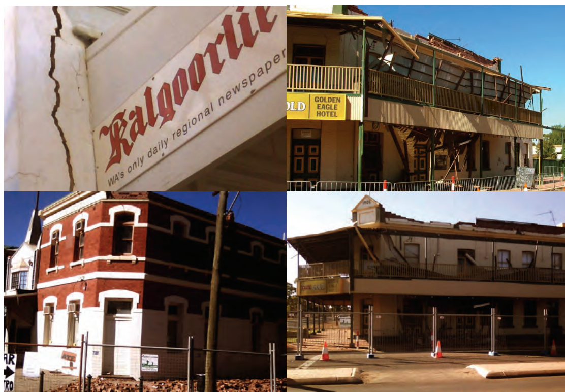
Figure 17: Building damage caused by the 20th April earthquake.
