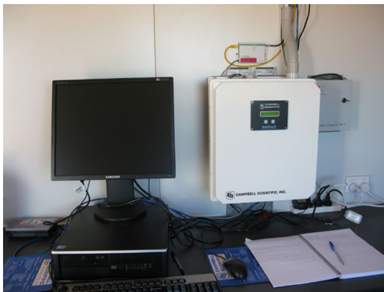
Figure 11: Environmental enclosure cabinet for the weather station mounted on the wall in the container next to the supervisor PC
