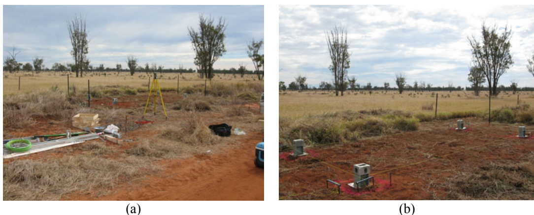
Figure 12: (a) Mapping out the location of the container showing a surveyor's level; (b) positions of cement pads
