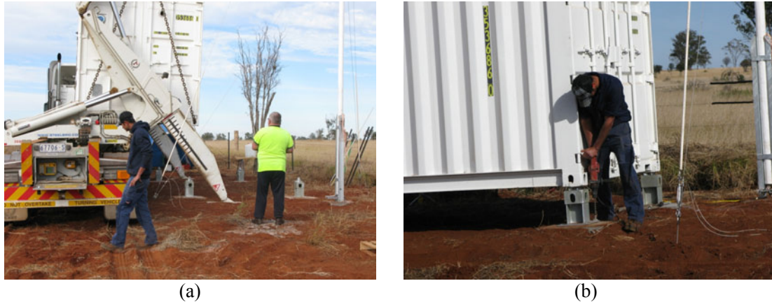
Figure 15: (a) Crane truck lifting container to position on footings; (b) securing the container footings to concrete pads
