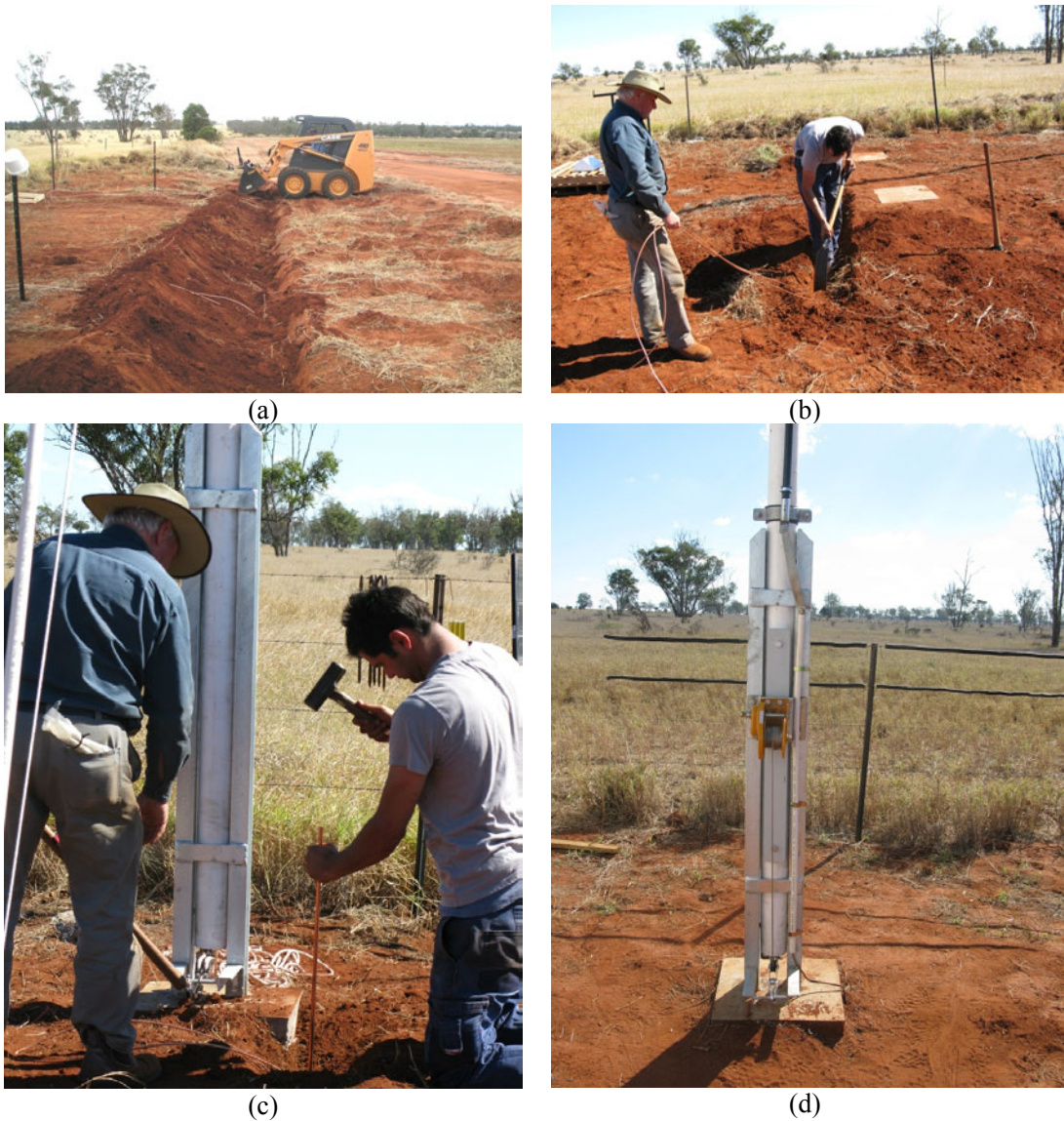
Figure 14: Installing the earth mat. (a) Bobcat used to drill holes and dig trench; (b) burying earth leakage wires; (c) hammering in 1.5m long copper coated steel rods; mast lightning arrester connected to earth mat (note pulley block replaced with winch)
