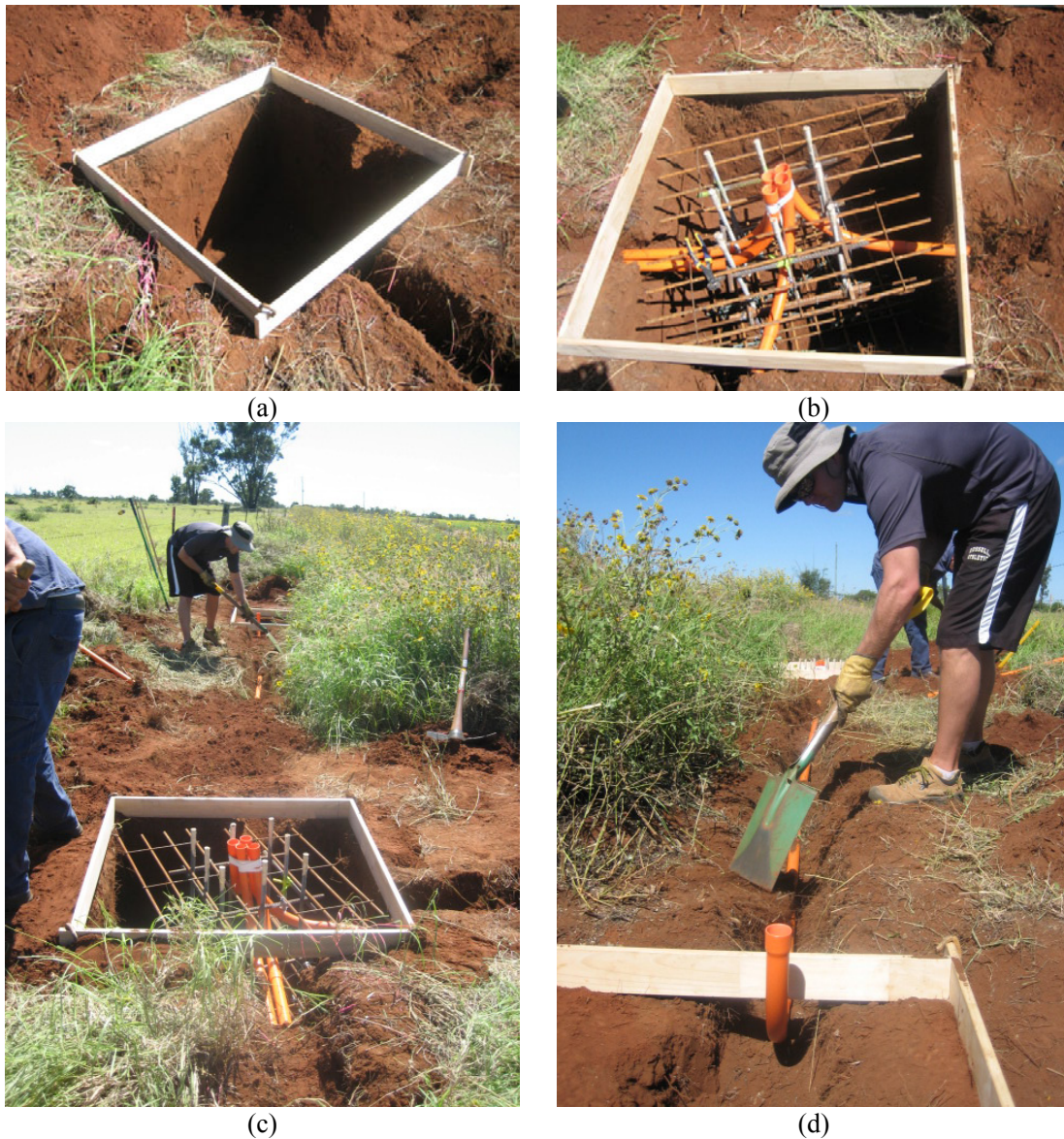
Figure 19: (a) Wooden frame for solar panel base; (b) frame for tower with conduits for power and earth leakage; (c) tower base (foreground) and solar panel base (rear); (d) conduit for power from solar panels to tower
