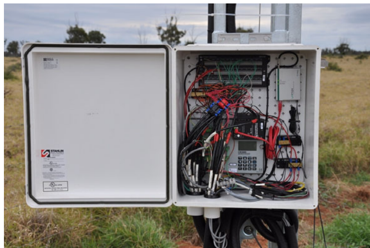
Figure 26: Wiring for EC tower
