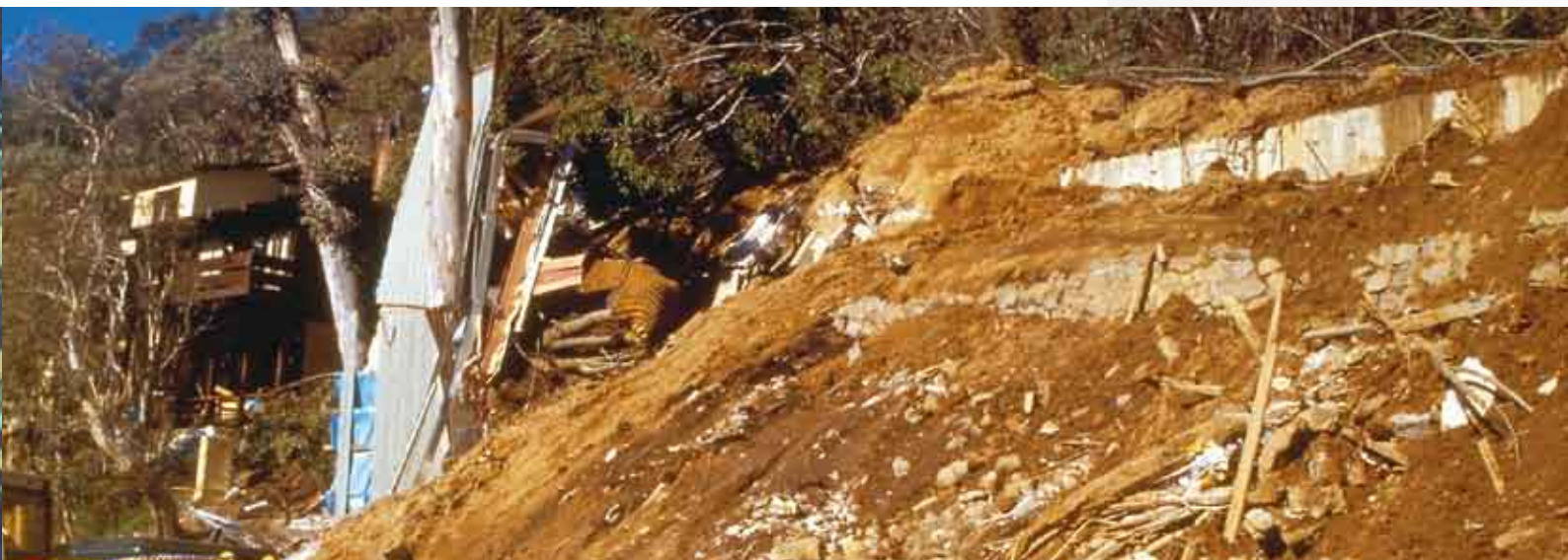
Side view of a fatal landslide at Thredbo, New South Wales, July 1997 Photo courtesy: Geoscience Australia.
