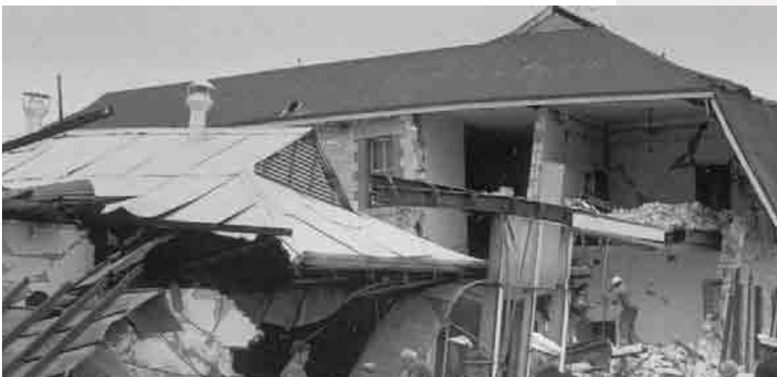
A collapsed house following an earthquake in Meckering, Western Australia, October 1968 Photo courtesy: Emergency Management Australia.
