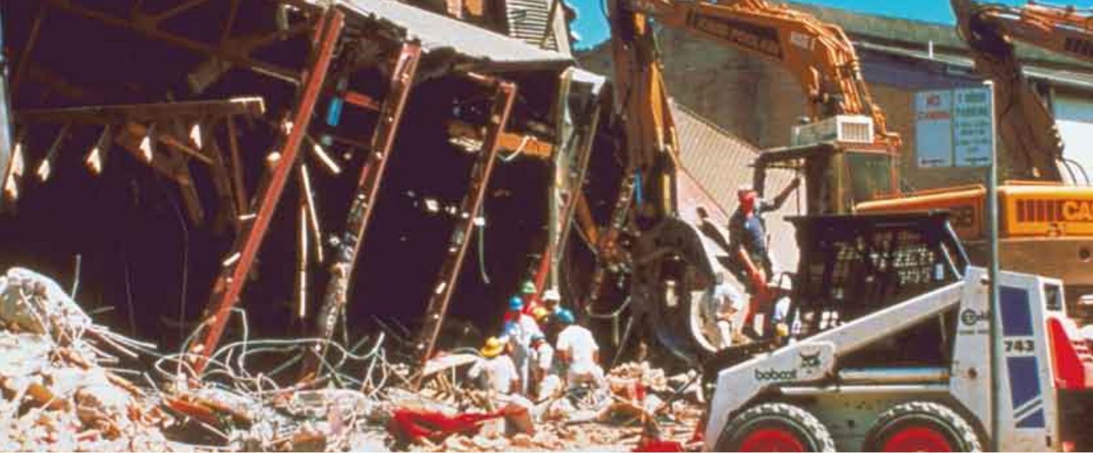
Damage sustained to the Workers Club following an earthquake in Newcastle, New South Wales, December 1989 Photo courtesy: Emergency Management Australia.
