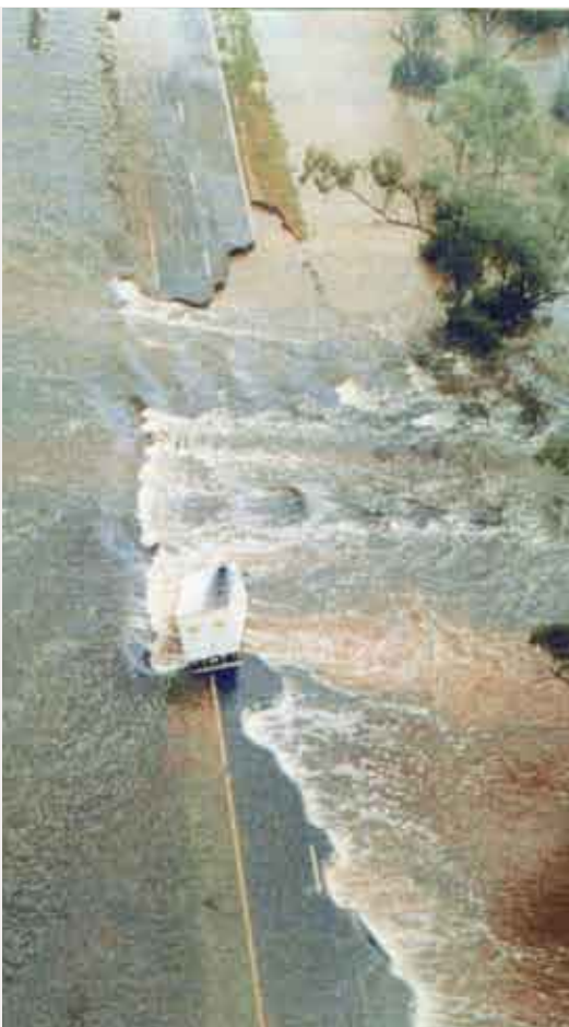
Flood damage to the Mitchell Highway near Nyngan, New South Wales, April 1990 Photo courtesy: Emergency Management Australia.
