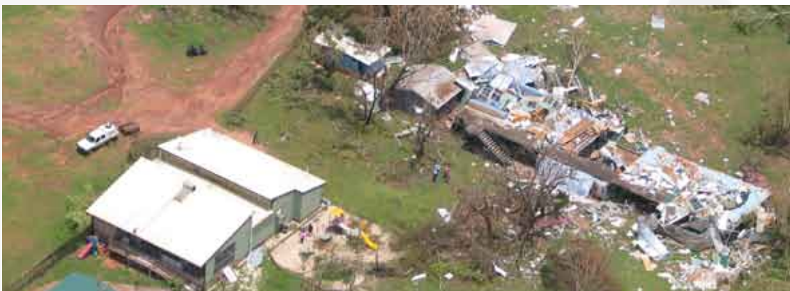
Damage to the Minjilang community school caused by Cyclone Ingrid on Croker Island, Northern Territory, March 2005 Photo courtesy: Bureau of Meteorology/Bill Milne.
