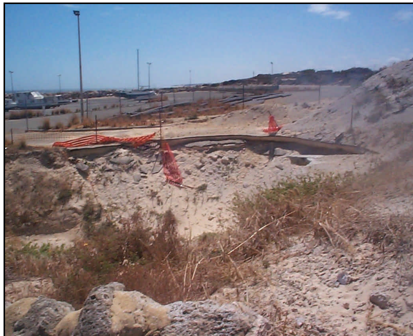
Figure 3.16 Road collapse in Holocene limestone at Two Rocks
