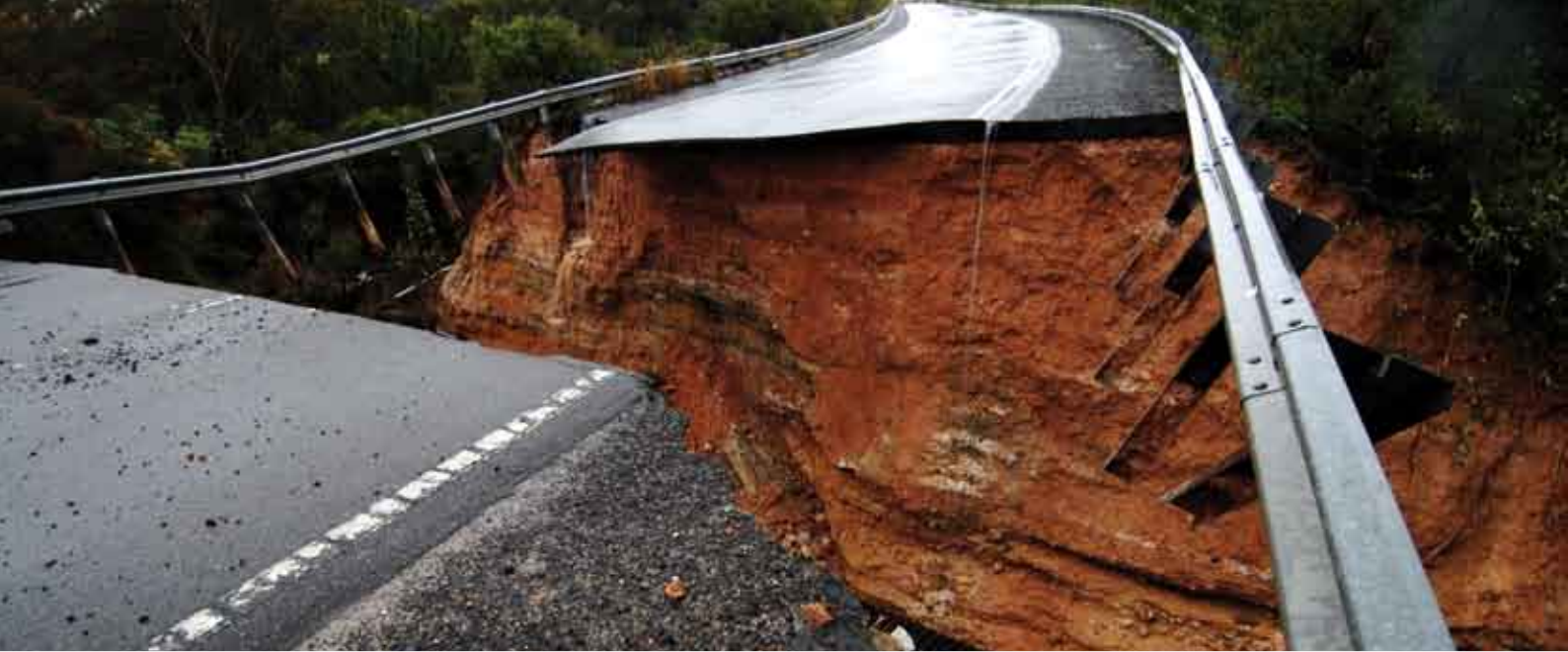
The collapsed part of the road along the Old Pacific Highway following a severe storm near Somersby in the central coast region, New South Wales, June 2007 Photo courtesy: AAP Image/Dean Lewins.
