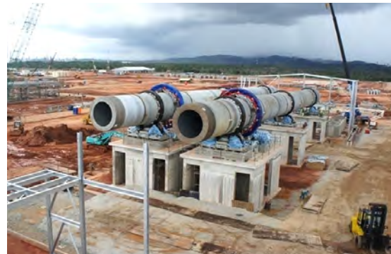
Figure 1.14. Installation of rotary kilns, Mount Weld Project, Malaysia. Photographs provided by Georgia Bunn (Lynas Corporation Limited: http://www.lynascorp.com/ )
