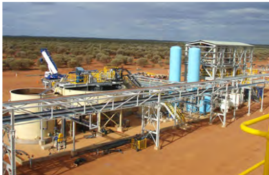
Figure 1.13. Filer press and thickener area at concentration plant, Mount Weld Project, Western Australia. Photographs provided by Georgia Bunn (Lynas Corporation Limited: http://www.lynascorp.com/ )
