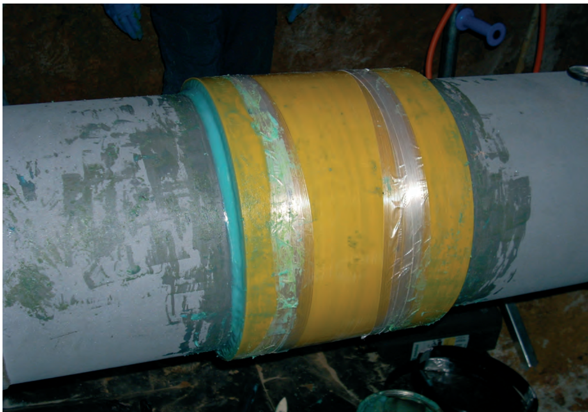
Figure 28: Pipeline fracture arrestor
