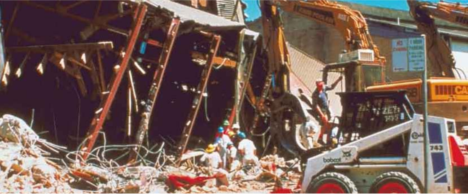
Damage sustained to the Workers Club following an earthquake in Newcastle, New South Wales, December 1989 Photo courtesy: Emergency Management Australia.
