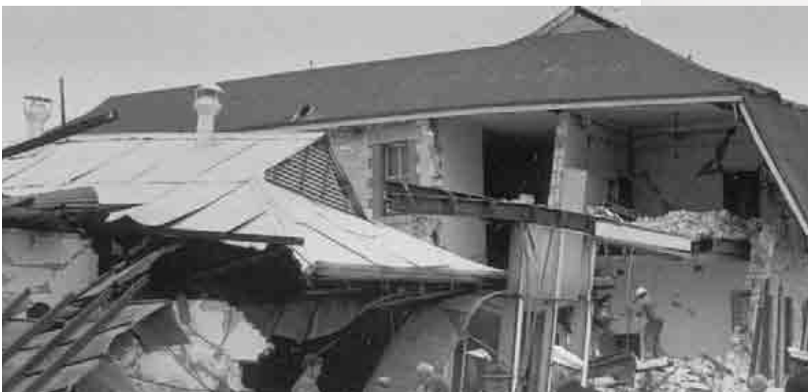
A collapsed house following an earthquake in Meckering, Western Australia, October 1968 Photo courtesy: Emergency Management Australia.
